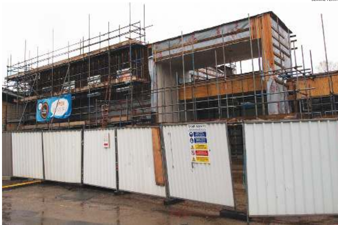
The renovated YUSU Student Centre was scheduled for initial completion by Christmas, but it has faced delays
